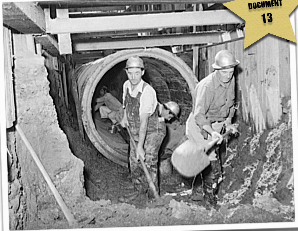
MEN WORK ON AN UNDERGROUND SEWER PIPE LINE SYSTEM IN SAN DIEGO, CALIFORNIA IN 1936
