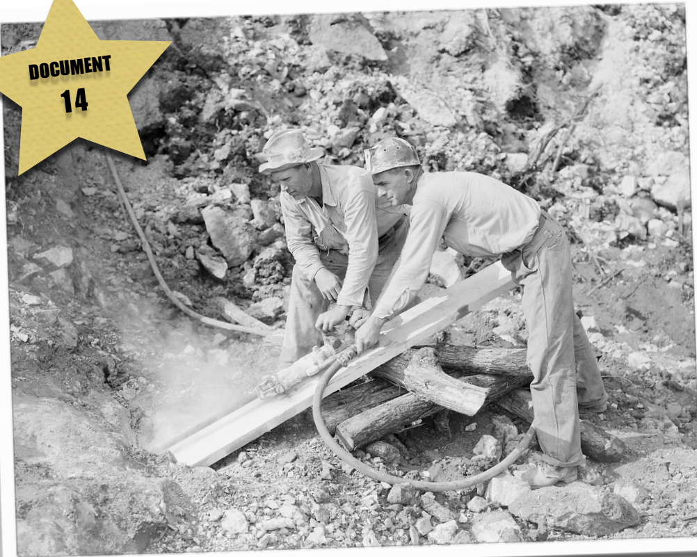
TWO MEN USE A HIGH-POWERED DRILL TO CRACK A BOULDER IN A ROADWAY DURING THE CONSTRUCTION OF NORRIS DAM IN TENNESSEE IN 1934
